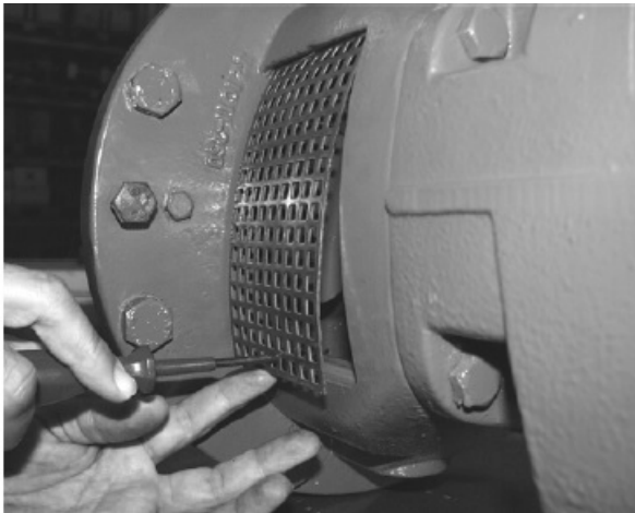
Figure 8: Motor lantern screen removal
